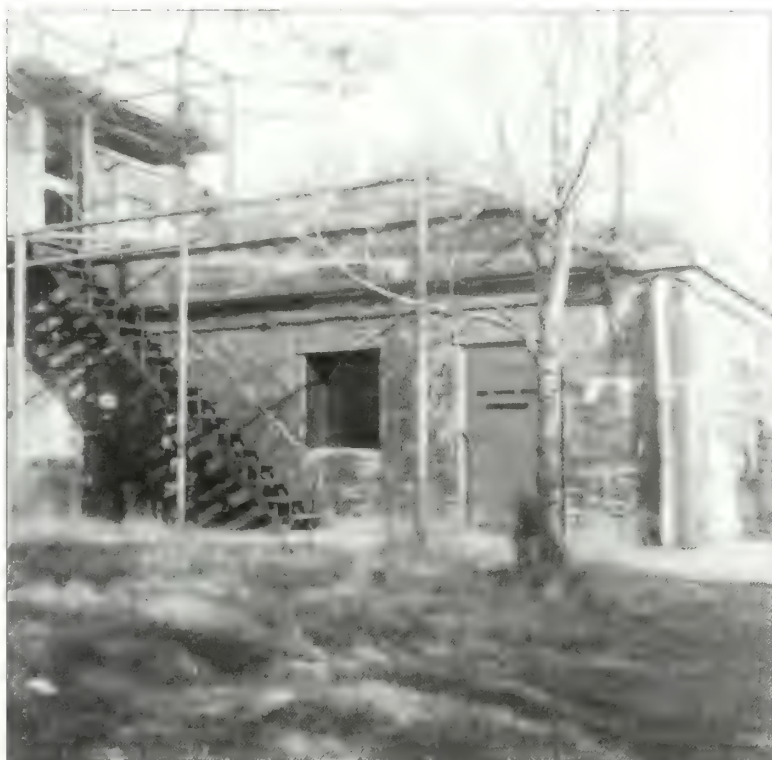
Figure 4.14. View looking northeast at central structure, Battery Gunnison, 1956. A tree appears west of the central structure and today, eight trees are located west of the battery in a staggered arrangement (GATE 11217).
